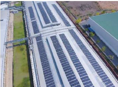
Solar Photovoltaic (PV) system at Shah Alam, Pulau Indah and Bentong plants, Malaysia with a total capacity of generating up to 10 MWp of energy.
