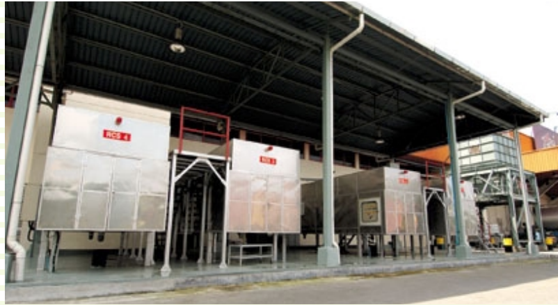
Organic waste conversion equipment at the Soft Drinks Shah Alam plant.
